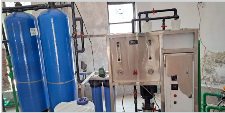
Water Filtration Plant
